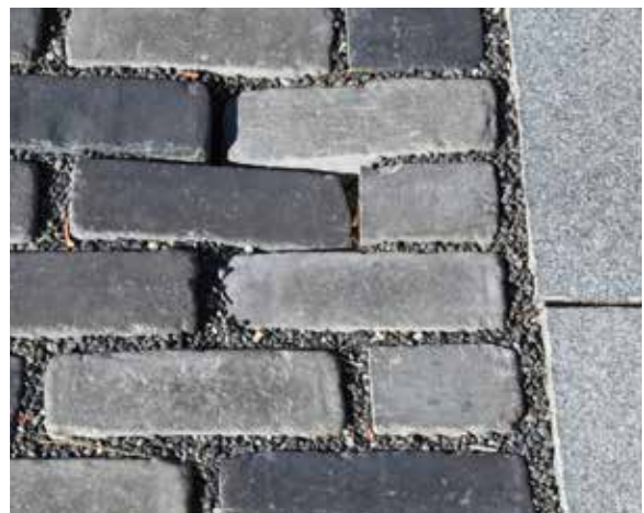
Example of washed out or settled joint material causing settlement.
